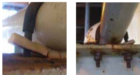
Failed I-Rod® imitations.
