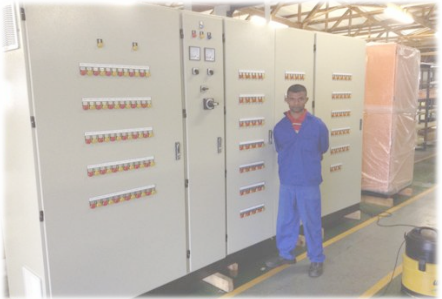
THS supplied Heat Trace Distribution Board No 1 of 2 – Lamson TLDD Project
